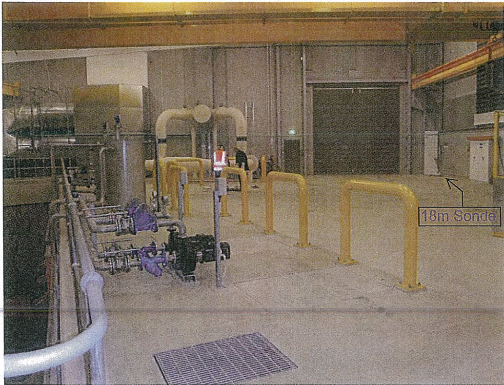
18m From Shaft - Orakei Domain Pumpstation (PS64) - 14/07/11
