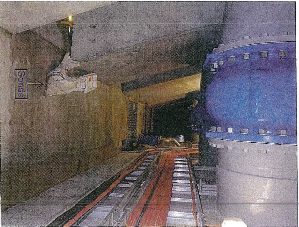
Below Pump #2 - Orakei Domain Pumpstation (PS64) - 14/07/11
